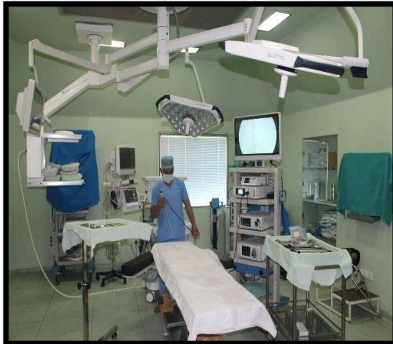
Modular Operation Theatre
